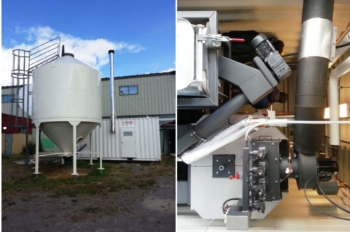
Figure 5: Nakzadil First Nation's biomass project heating the community centre.
